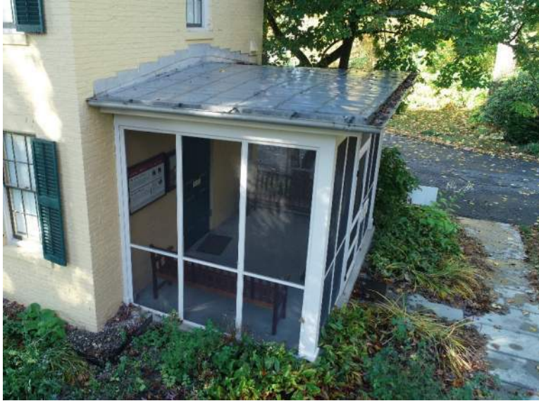
Figure 11: Entrance at north elevation, 2 steps at each doorway, with limited room between to install a ramp.
