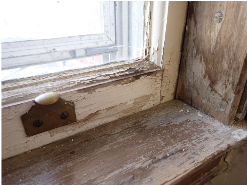
51. Second floor, west wall, detail of typical historic wood window deterioration
