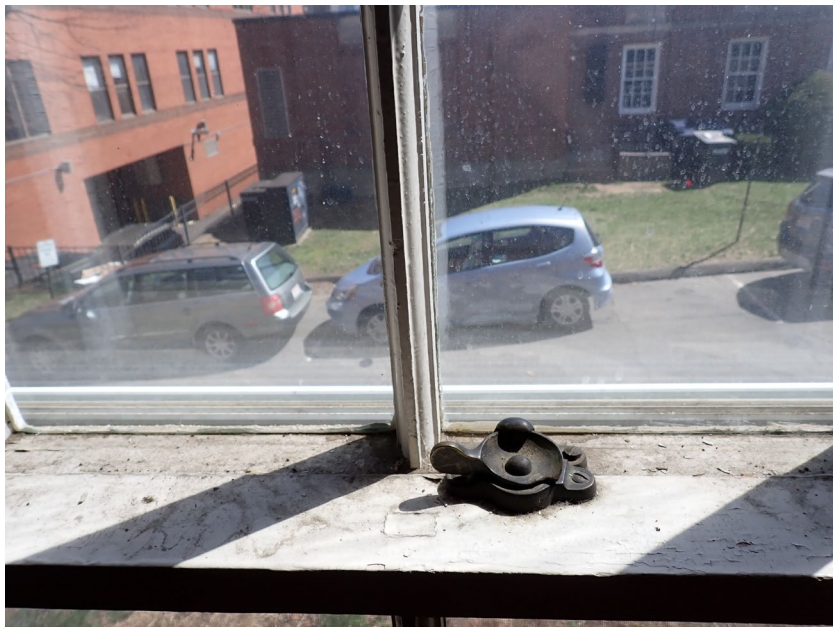
37. First floor, east wall, detail of typical historic wood window deterioration
