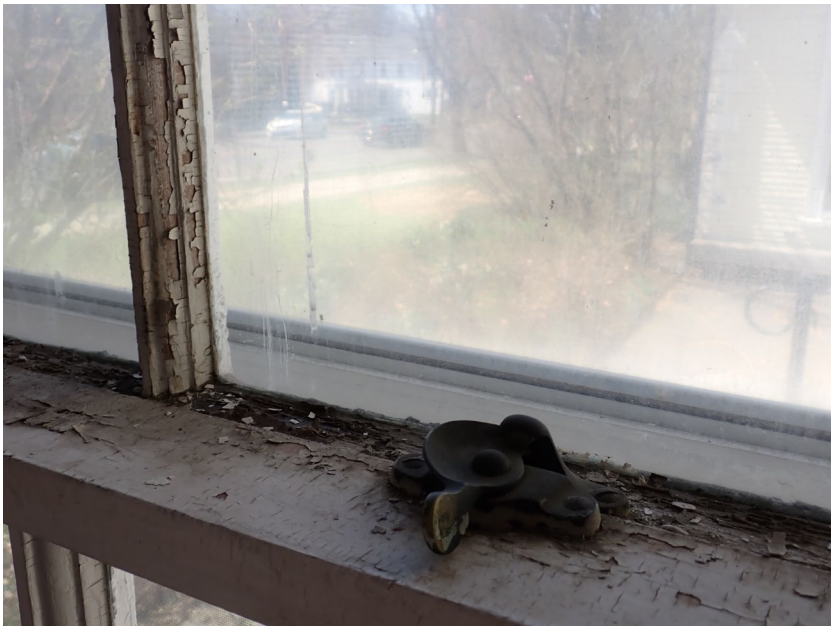
21. First floor, south wall, detail of typical historic wood window deterioration
