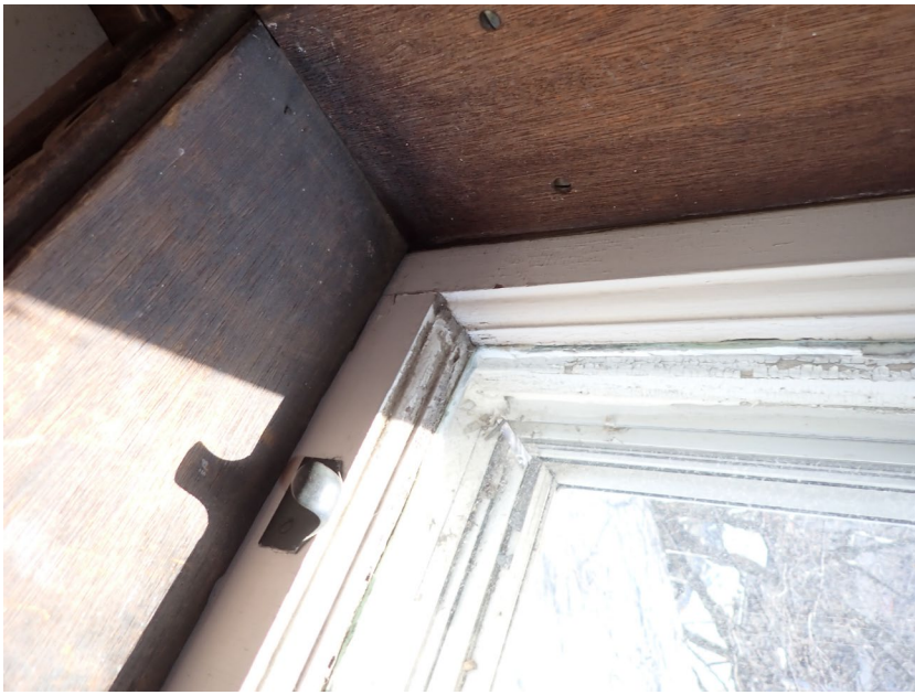
45. Second floor, south wall, detail of typical historic wood window deterioration
