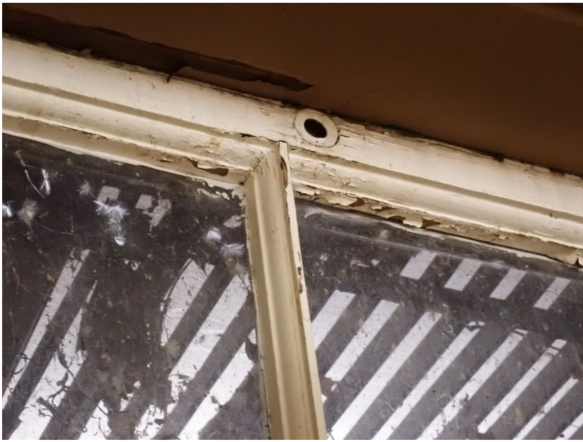
13. Basement level, south wall, detail of typical historic wood window deterioration
