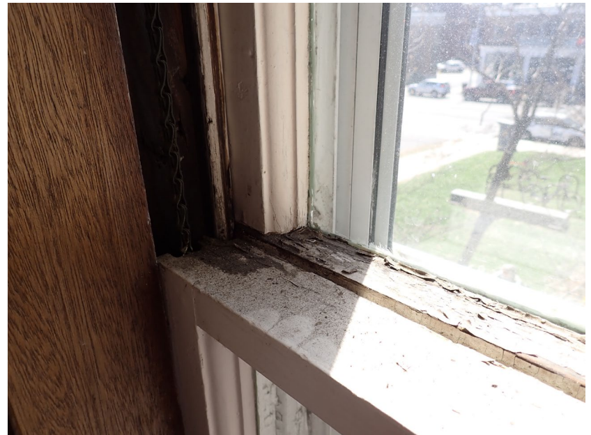
40. Second floor, south wall, detail of typical historic wood window deterioration
