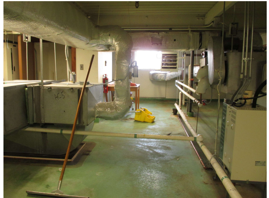
164. Third floor, mechanical room, view east
