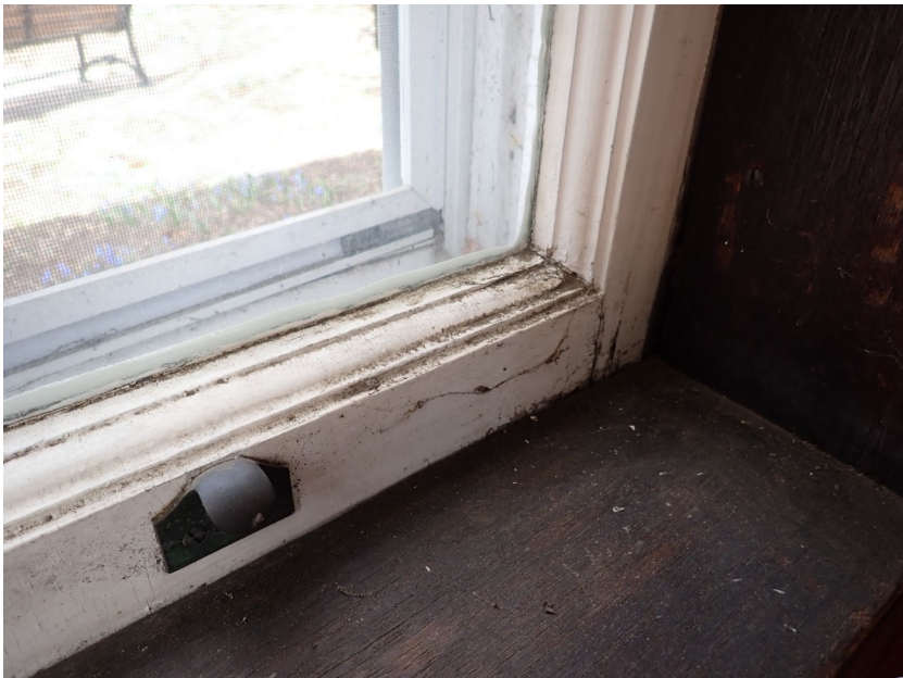
23. First floor, west wall, detail of typical historic wood window deterioration
