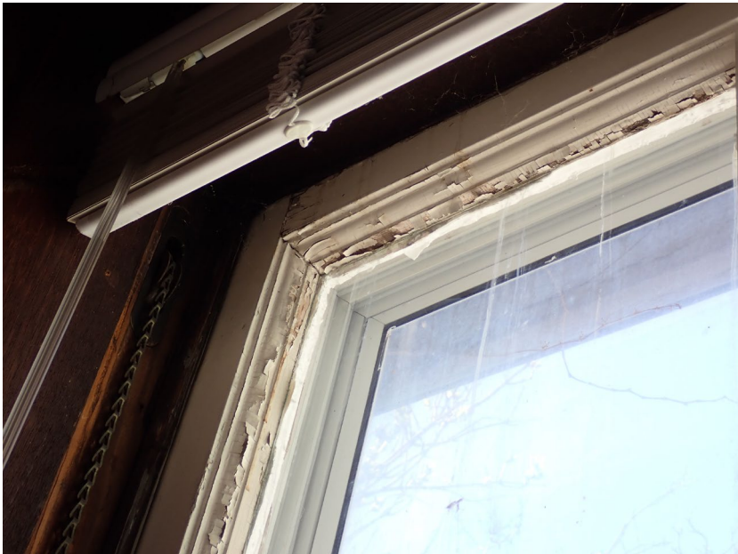
19. First floor, south wall, detail of typical historic wood window deterioration
