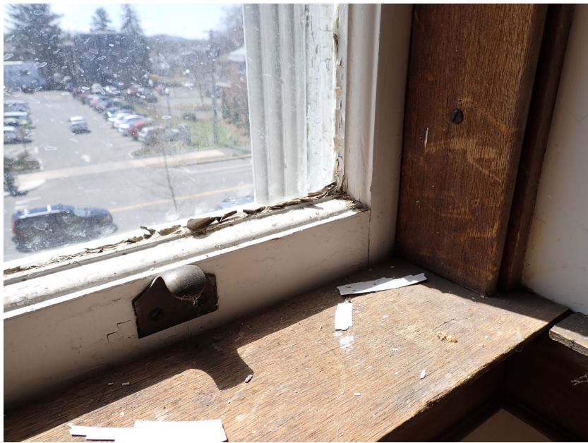
65. Third floor, south wall, detail of typical historic wood window deterioration
