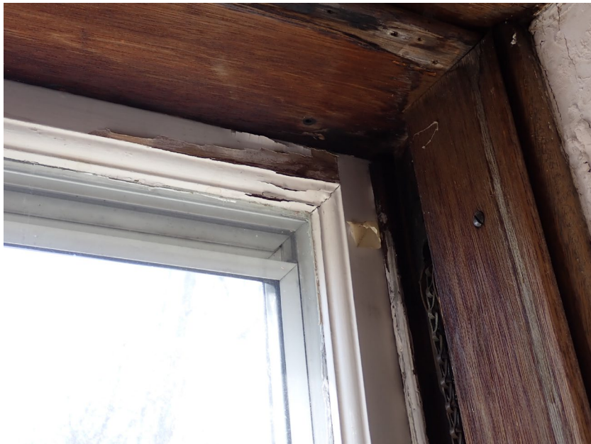
41. Second floor, south wall, detail of typical historic wood window deterioration
