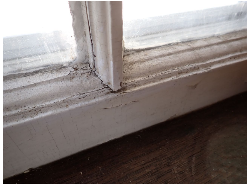
18. First floor, south wall, detail of typical historic wood window deterioration
