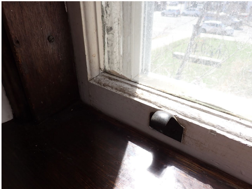
39. Second floor, south wall, detail of typical historic wood window deterioration
