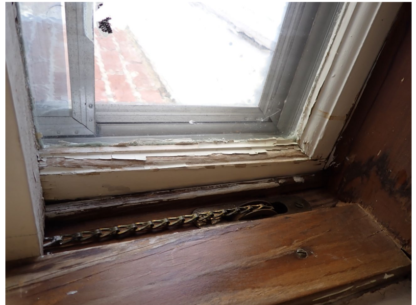
52. Second floor, west wall, detail of typical historic wood window deterioration
