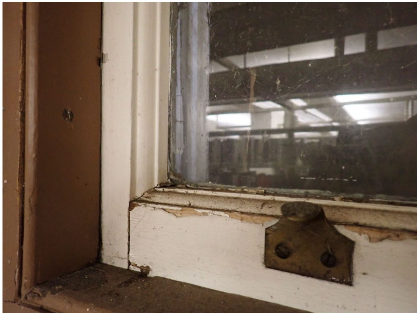
11. Basement level, south wall, detail of typical historic wood window deterioration
