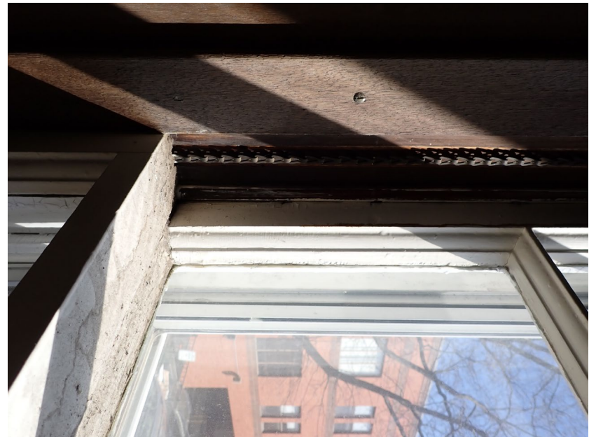
36. First floor, east wall, detail of typical historic wood window deterioration
