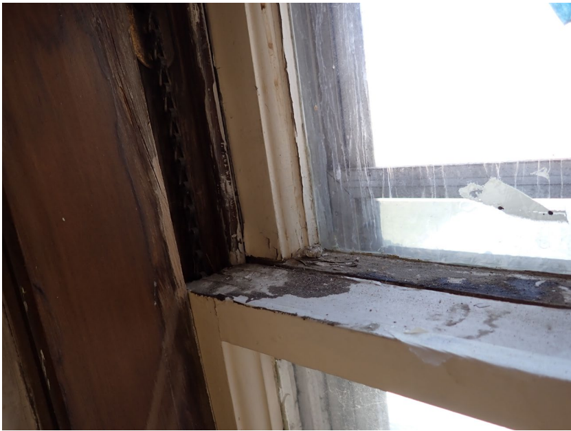
53. Second floor, west wall, detail of typical historic wood window deterioration
