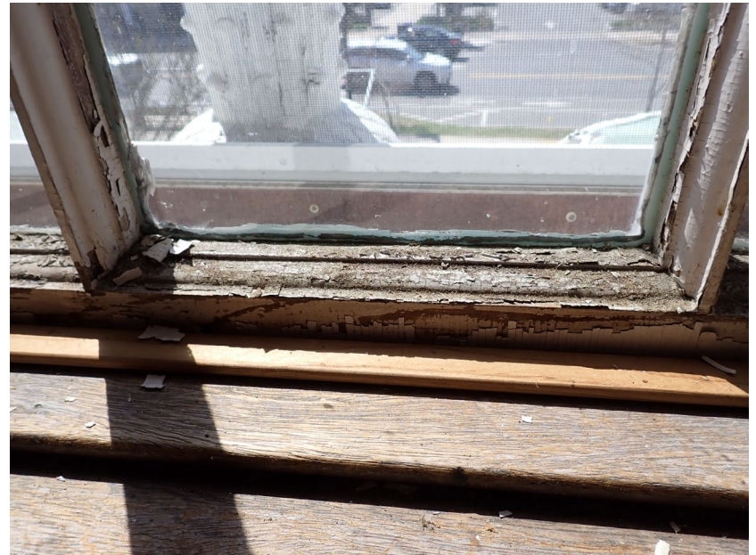
48. Second floor, south wall, detail of typical historic wood window deterioration
