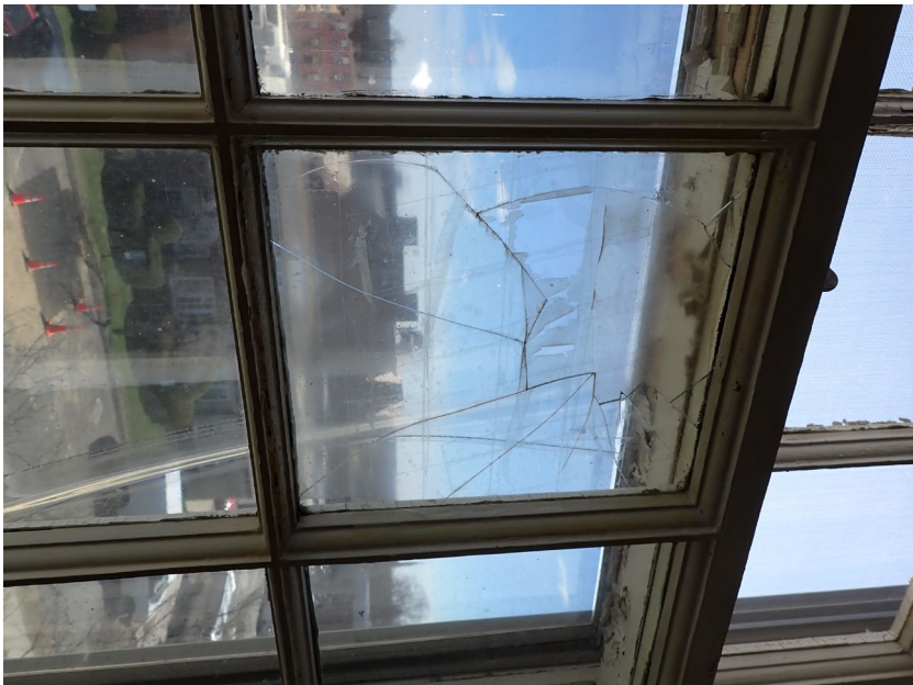
55. Third floor, east wall, detail of typical historic wood window deterioration
