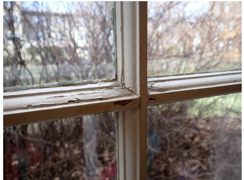
28. First floor, west wall, detail of typical historic wood window deterioration
