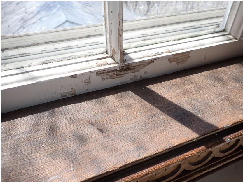
43. Second floor, south wall, detail of typical historic wood window deterioration
