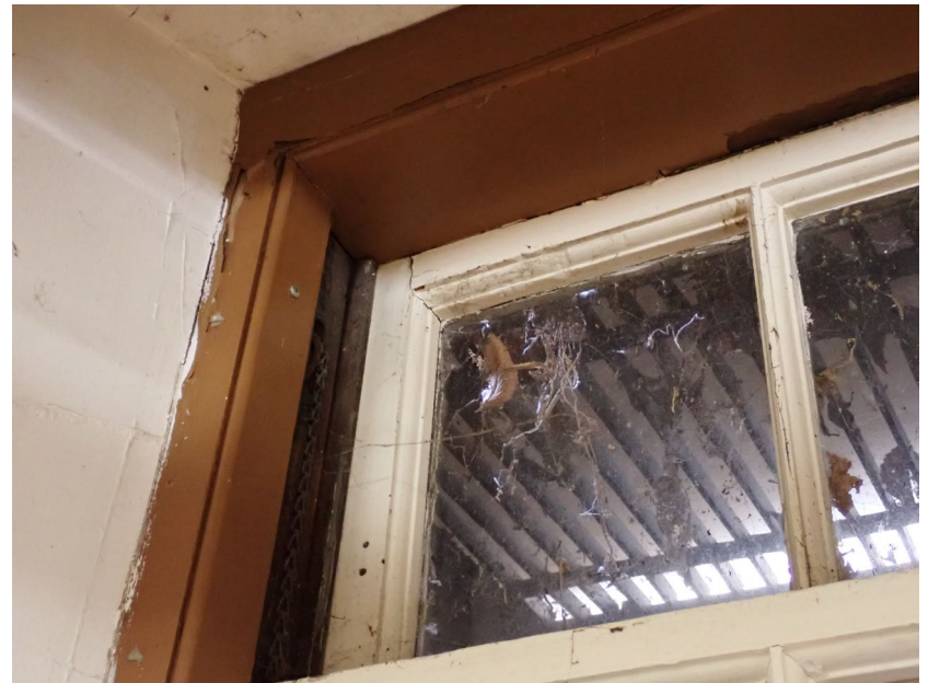
12. Basement level, south wall, detail of typical historic wood window deterioration
