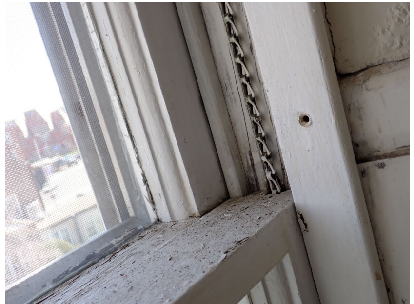
56. Third floor, east wall, detail of typical historic wood window deterioration
