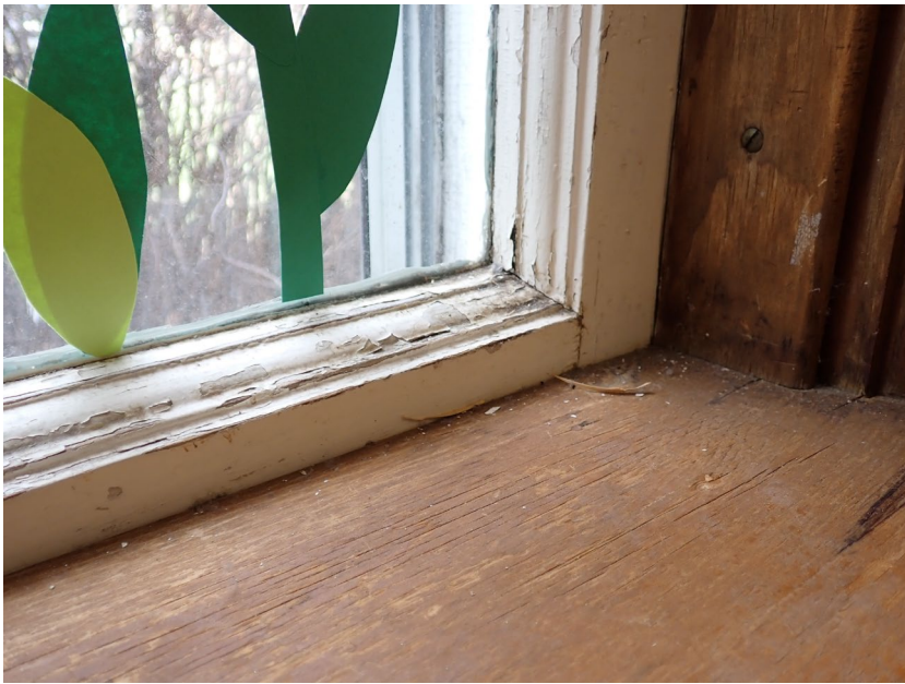
29. First floor, west wall, detail of typical historic wood window deterioration
