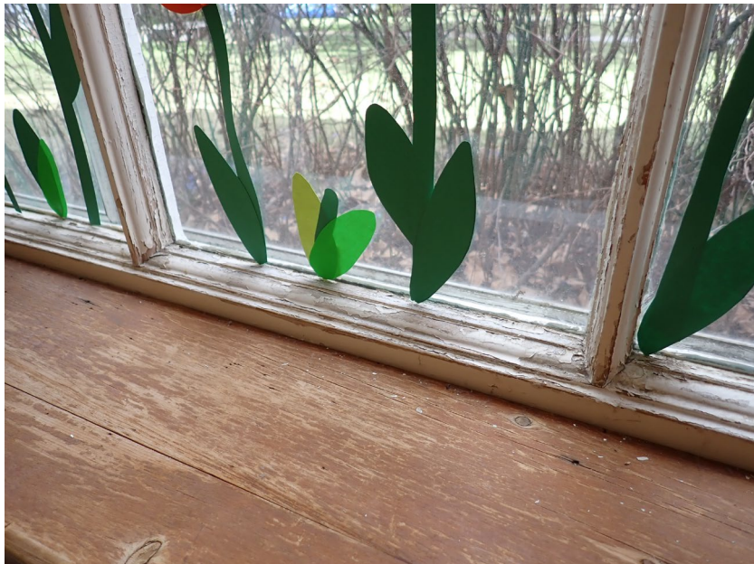
27. First floor, west wall, detail of typical historic wood window deterioration
