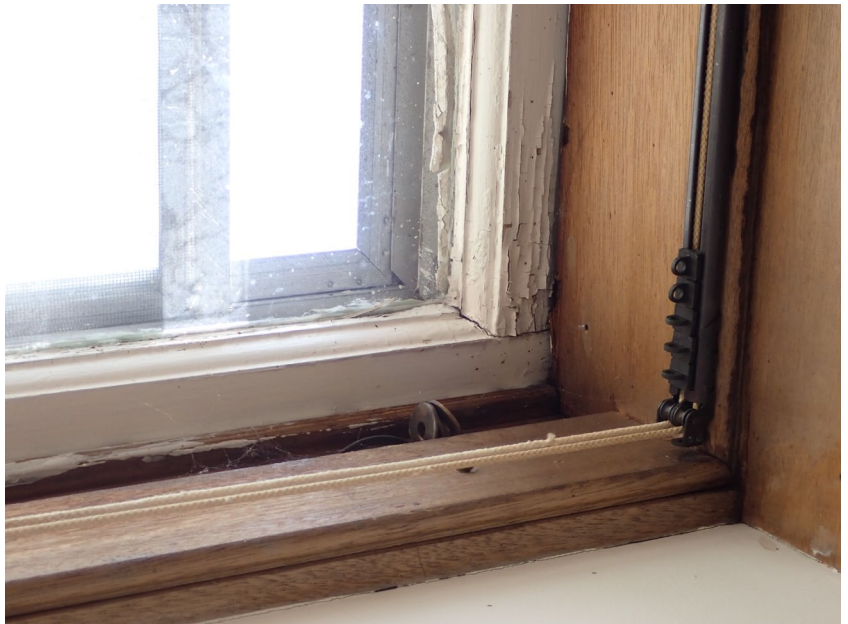
64. Third floor, south wall, detail of typical historic wood window deterioration
