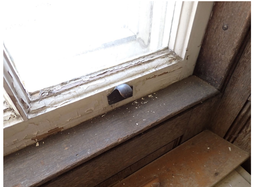
34. First floor, east wall, detail of typical historic wood window deterioration
