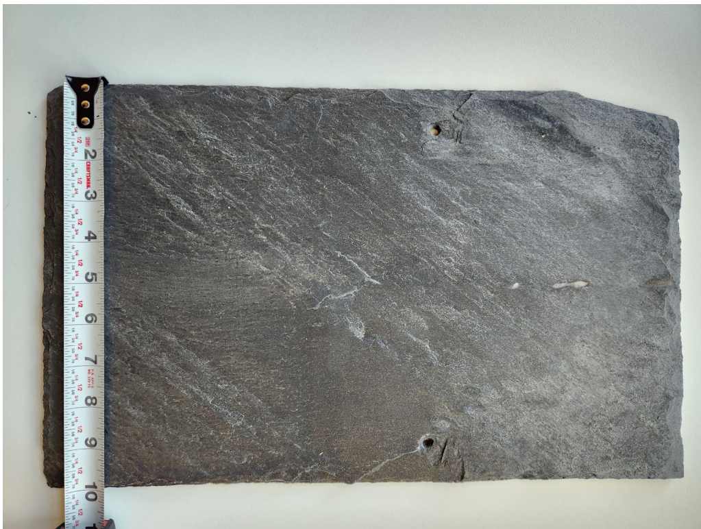
2. Salvaged historic Buckingham slate, typical condition
