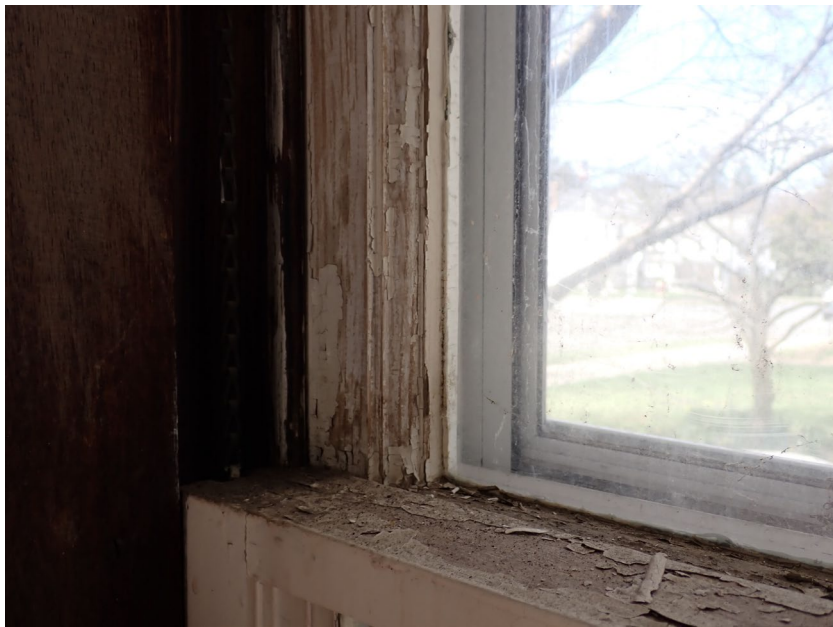
25. First floor, west wall, detail of typical historic wood window deterioration
