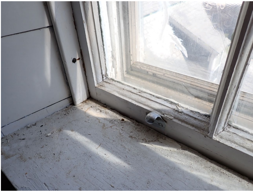
57. Third floor, east wall, detail of typical historic wood window deterioration
