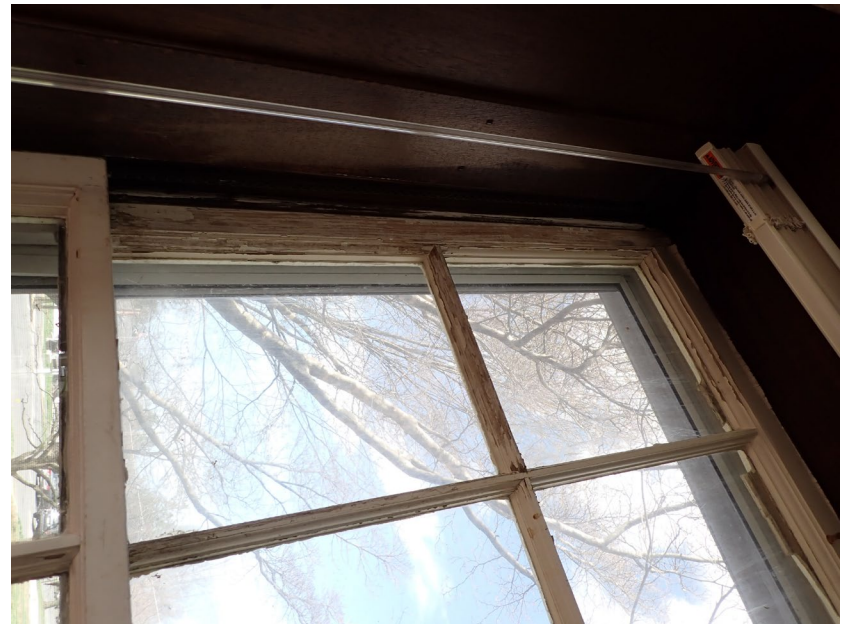
24. First floor, west wall, detail of typical historic wood window deterioration
