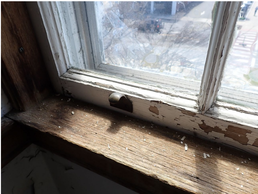
59. Third floor, south wall, detail of typical historic wood window deterioration
