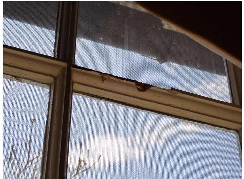
44. Second floor, south wall, detail of typical historic wood window deterioration
