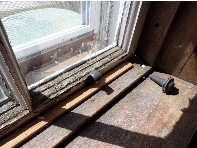
47. Second floor, south wall, detail of typical historic wood window deterioration
