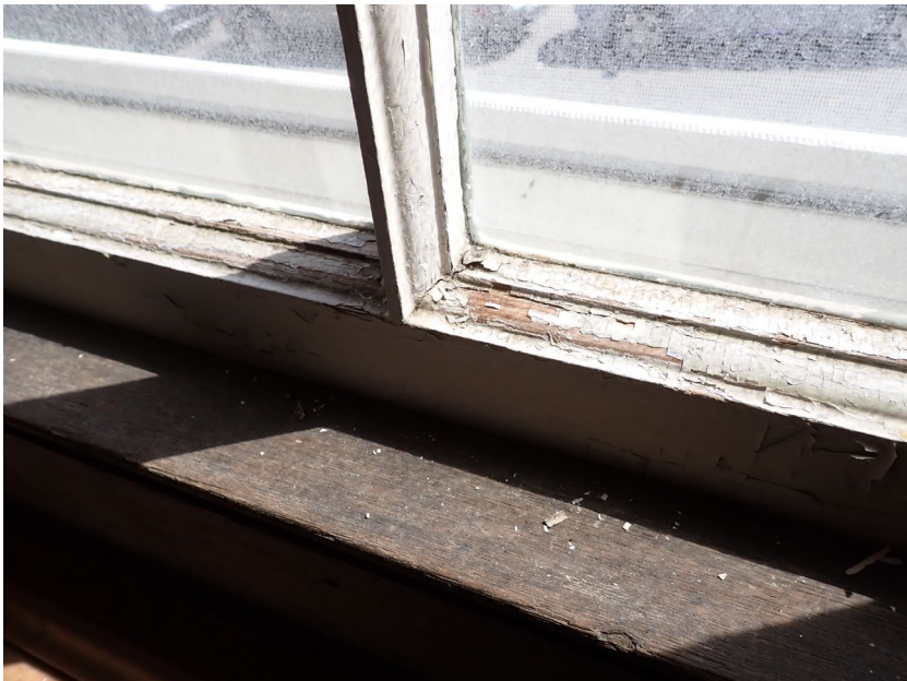
35. First floor, east wall, detail of typical historic wood window deterioration
