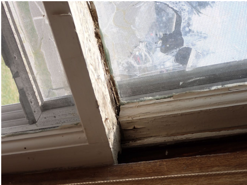
63. Third floor, south wall, detail of typical historic wood window deterioration
