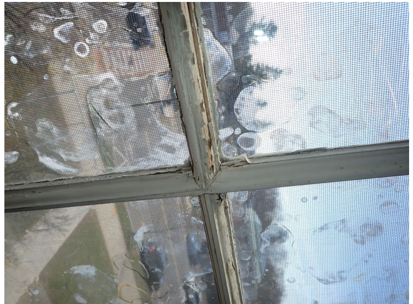
60. Third floor, south wall, detail of typical historic wood window deterioration
