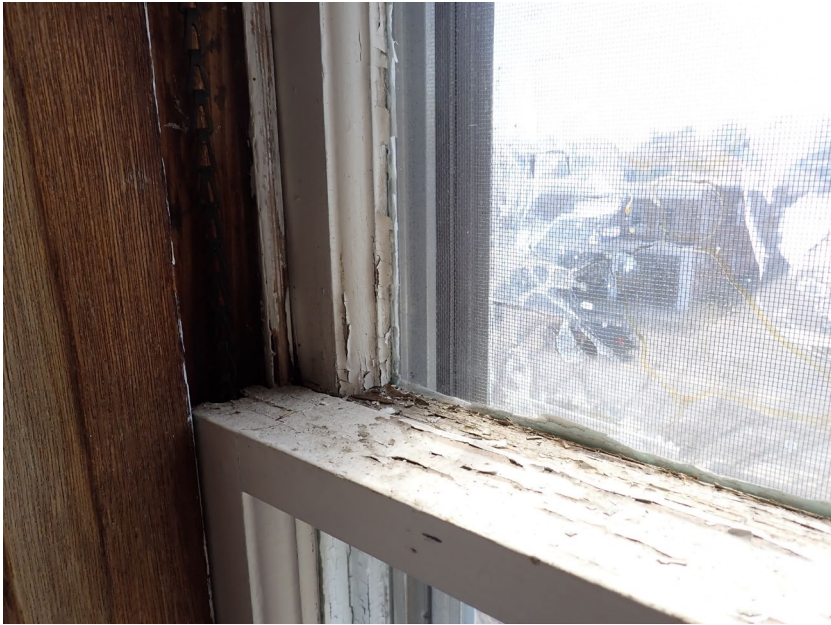
61. Third floor, south wall, detail of typical historic wood window deterioration
