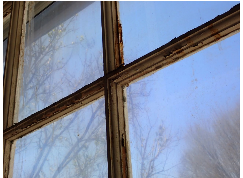
20. First floor, south wall, detail of typical historic wood window deterioration
