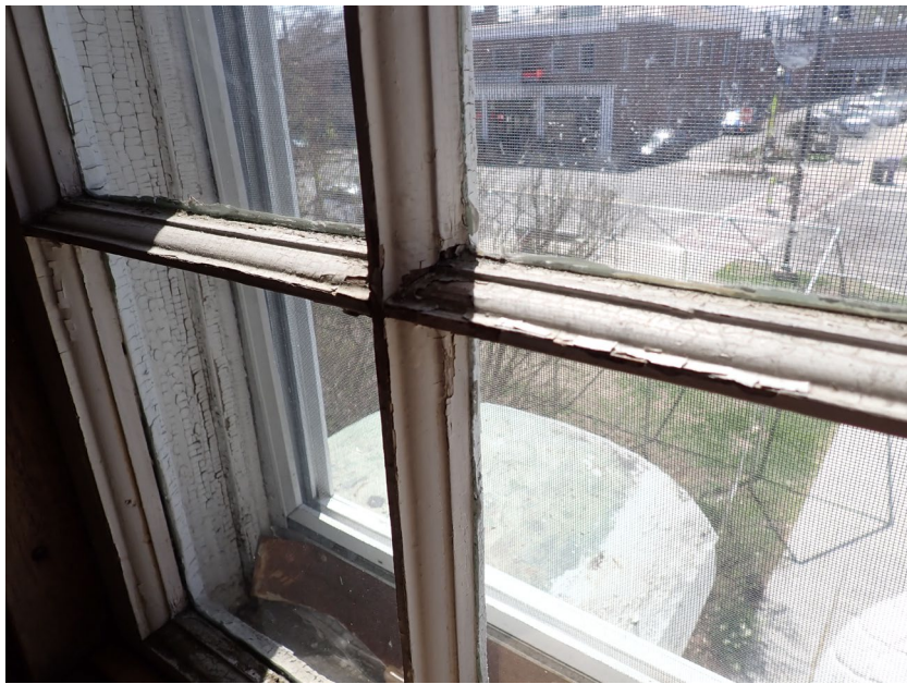
49. Second floor, south wall, detail of typical historic wood window deterioration
